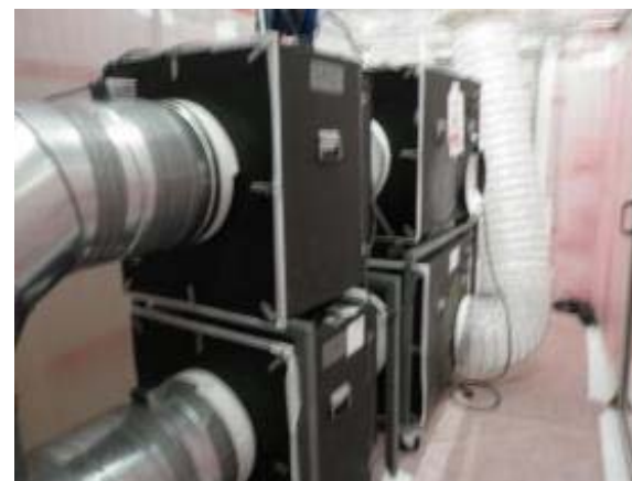
Ventilation with 2 lines of very high efficiency filters
